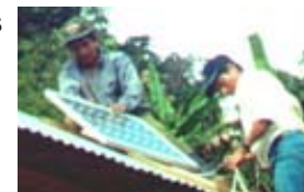
Most radio systems are solar powered.
